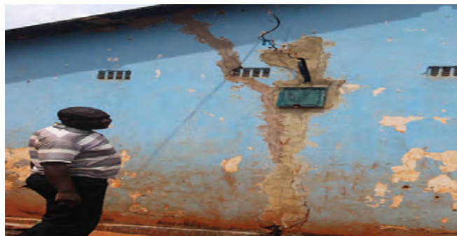
Figure 19: Kyafukuma Secondary School head teacher's House, possibly damaged by mine blasting.
