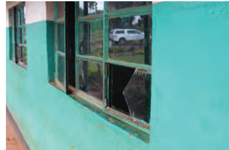
Figure 17: The windows of one of the classrooms at Kyafukuma Secondary School.
