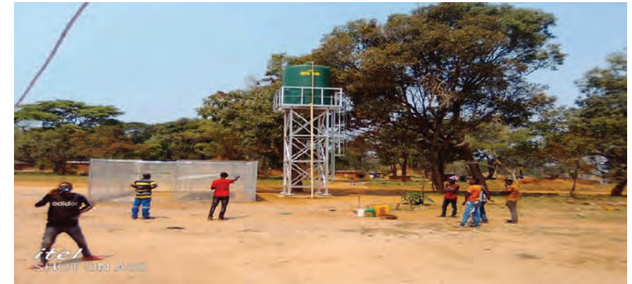
A mechanised borehole, solar powered with 10 000 -liter tank, constructed by the Consolidated Gold Company in Kasenseli. Source: Field Photo.
